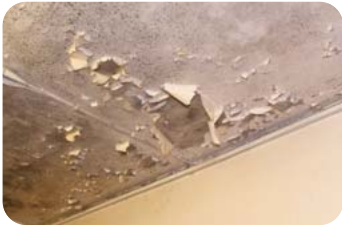
e.g. black spot mould growth on a ceiling
